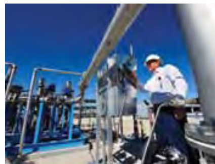
This Veolia DBO project in Tampa Bay is a state-of-the-art surface water treatment plant
